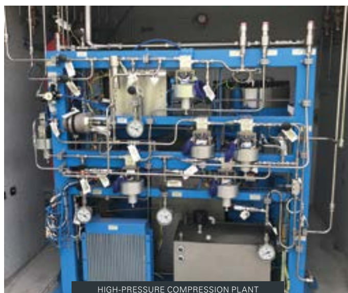
HIGH-PRESSURE COMPRESSION PLANT
